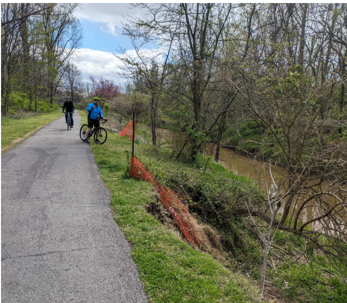
Figure 5.23- The stream bank above needs stabilization work before it undermines the trail.
