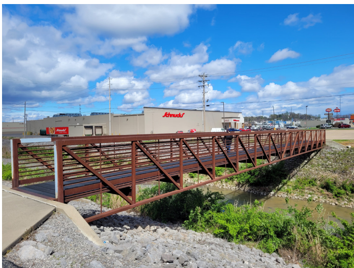
Figure 4.25 - Structures, such as bridges and walls are expensive and affect project feasibility.
