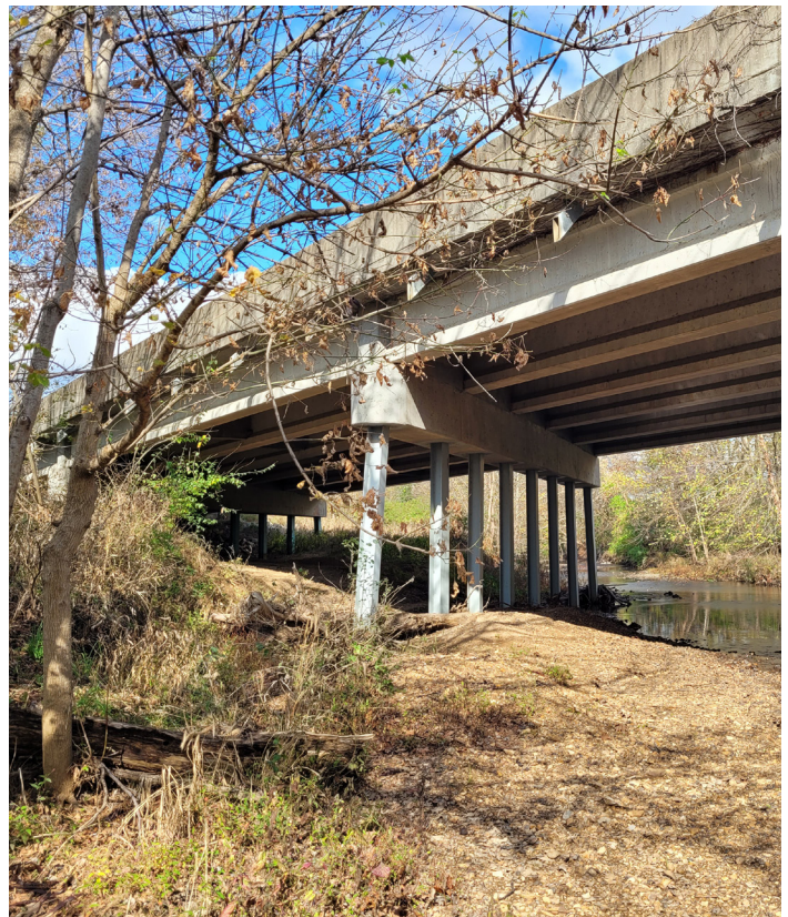
Figure 5.11 - The images above show there is lots of space for the trail to cross under Cape La Croix Road.
